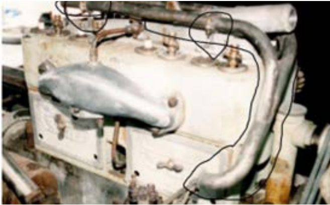
Ignition Wire Conduit & Support Brackets
