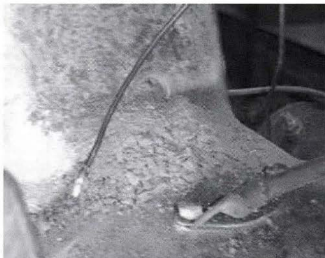
Rust and Scale in the Block
